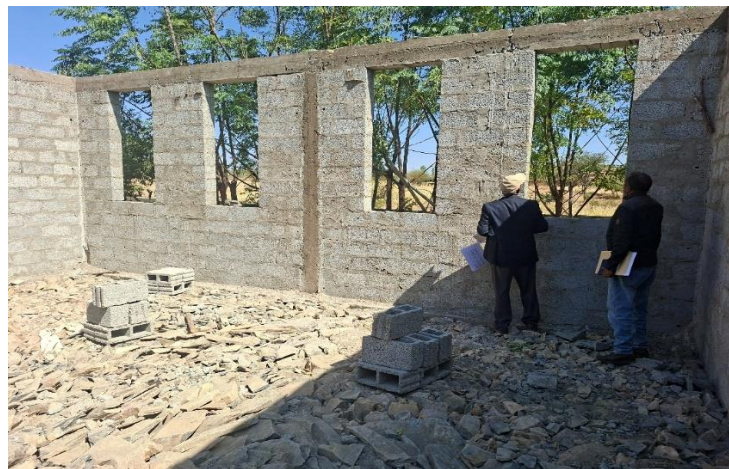
Figure 2: Back side classroom viewed from interior, top tie beam, column & hollow block masonry
